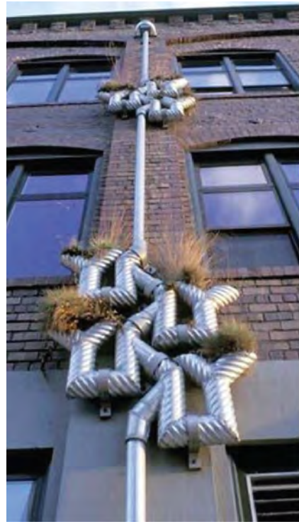
Visible Rooftop Rainwater Collection
